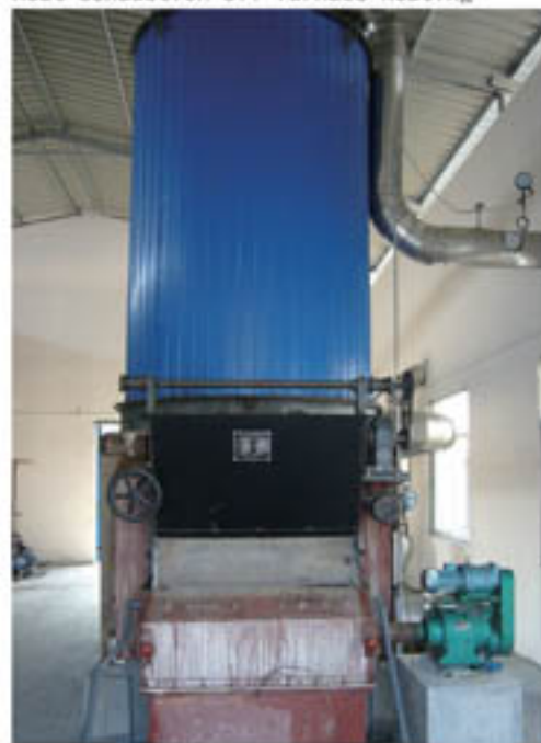
导热油炉供热系统 Heat conduction oil furnace heating
