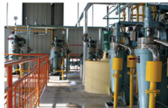
棉籽油连续精炼车间 Cottonseed oil continuous refining workshop
