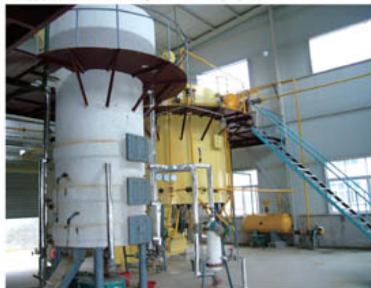
蒸脱系统 Desolventizing and toasting system
