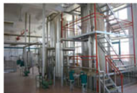
物理脱酸脱臭系统 Physical deacidification and deodorization system
