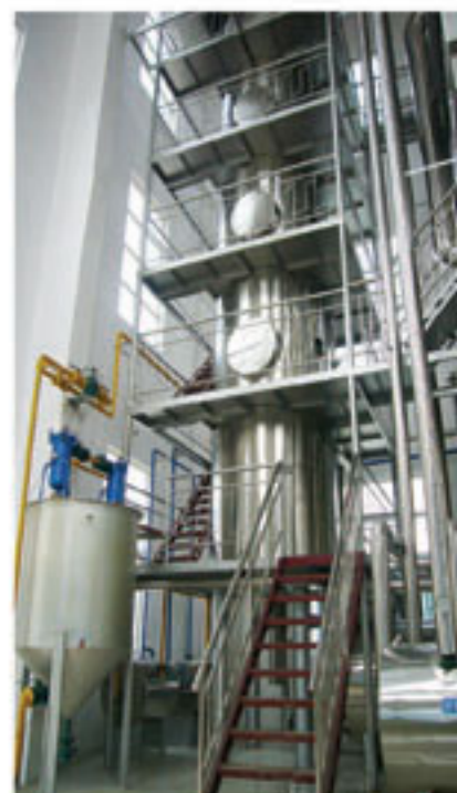
脱臭塔 Deodorization Tower
