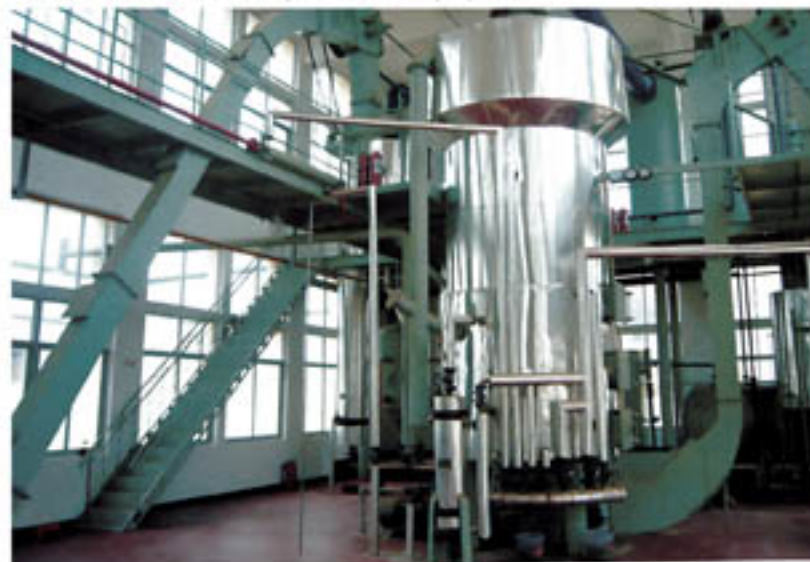
蒸脱系统 Desolventizing and toasting system
