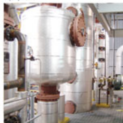
Evaporation and steam stripping equipment
