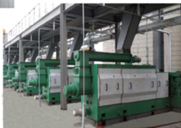
榨油工段 Oil pressing section
