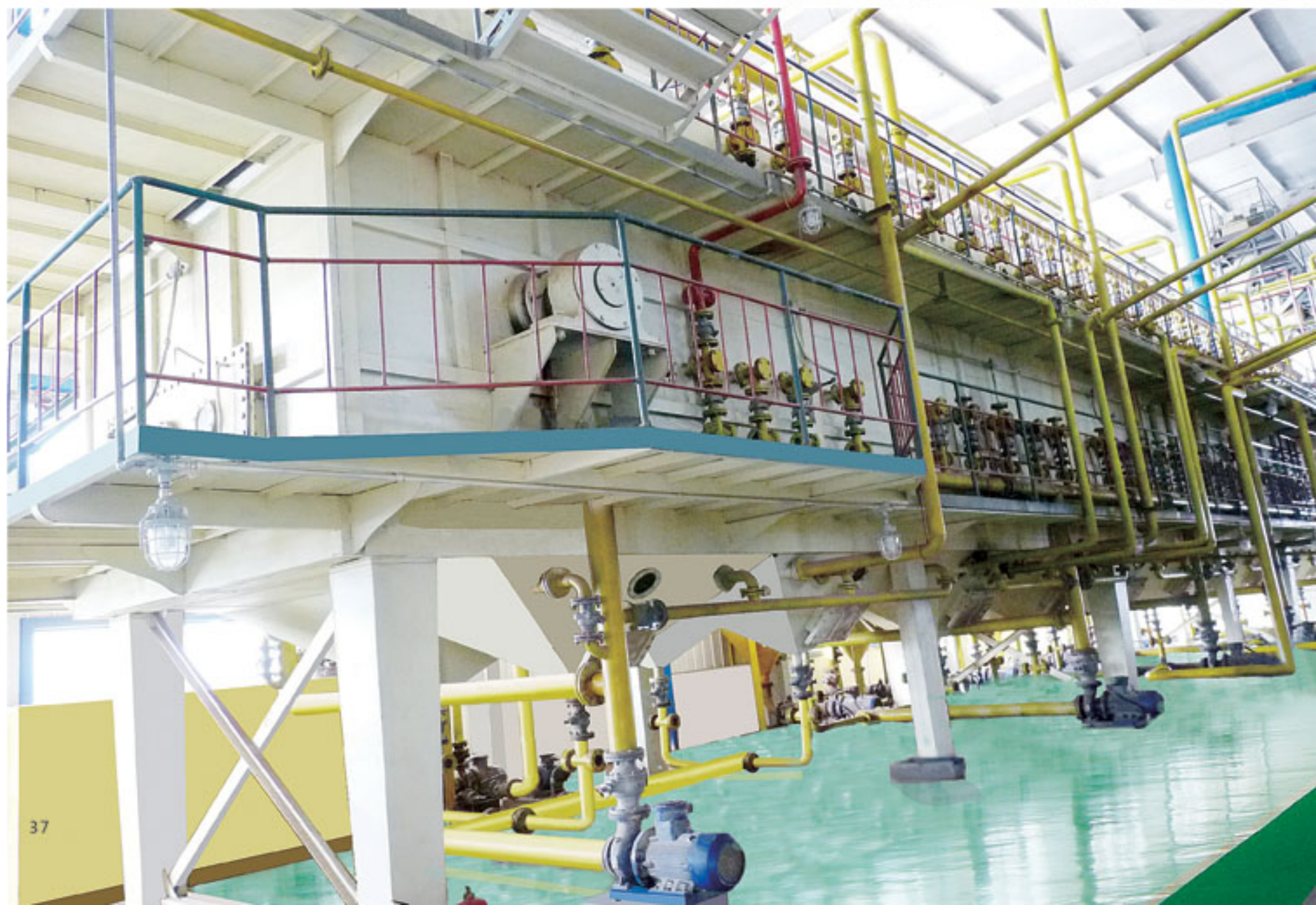
拖链浸出器 Towline extractor
